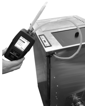
Fig. 69 - Digital pressure switch connection 1
