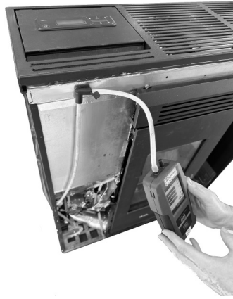
Fig. 57 - Digital pressure switch connection
