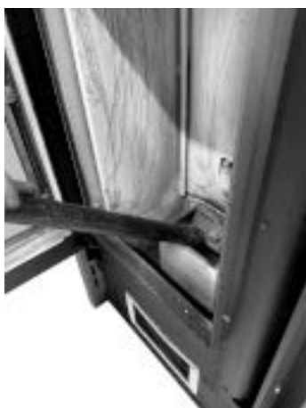
Fig. 35 - Burning pot box cleaning
