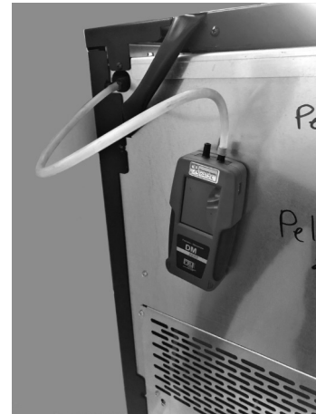
Fig. 33 - Digital pressure switch connection
